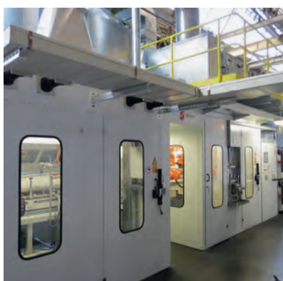
View on induction cabinet and paint booth
